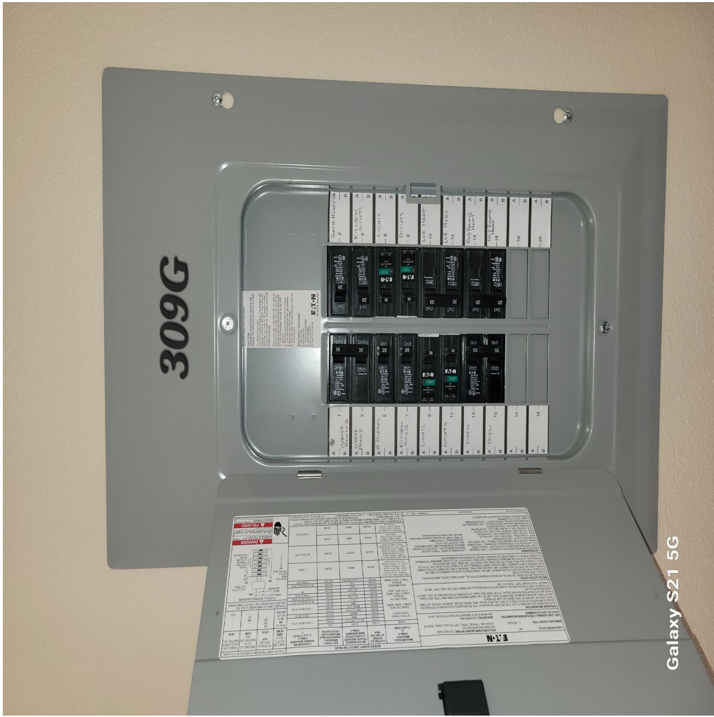
New Pushmatic Panel
