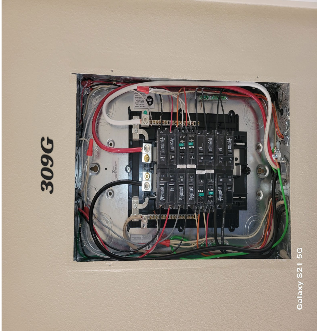
New Code Compliant Panel
